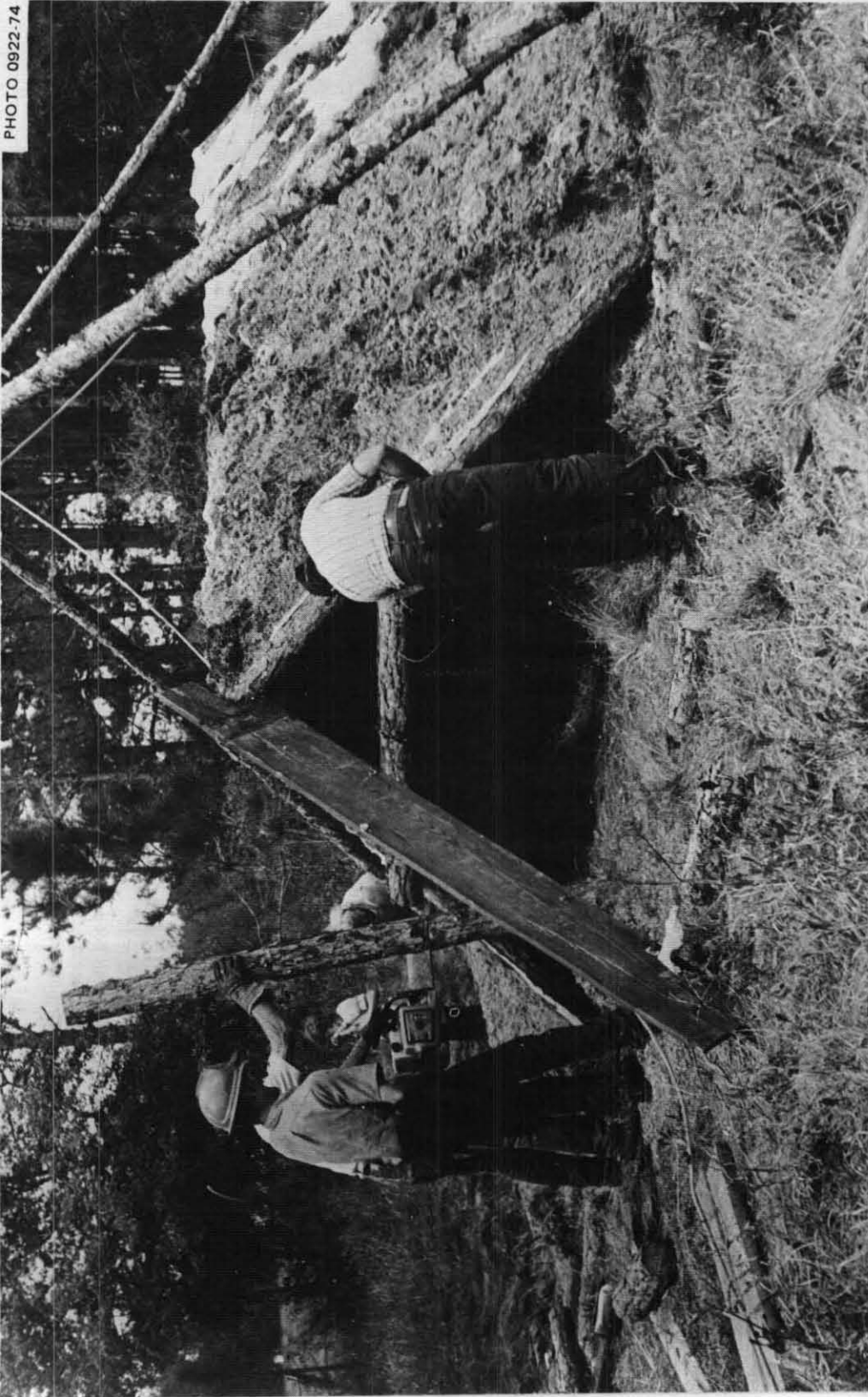
Fig. 5.49. Unnecessary work and delay resulted because these families failed to follow some of the instructions, especially as regards placing earth on the shelter starting from ground level and working upward. While Kearny was going to his car to get some food (the mud prevented his driving his station wagon to this site), the ridge of this shelter shifted lengthwise about 4 in. The builders stopped this move with the board brace pictured and then pulled the whole shelter back into its correct position with a chain and powerful hand-operated winch.
